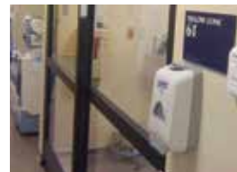
Automatic isolation room door with touchless system to ensure doors are only opened when activated.
